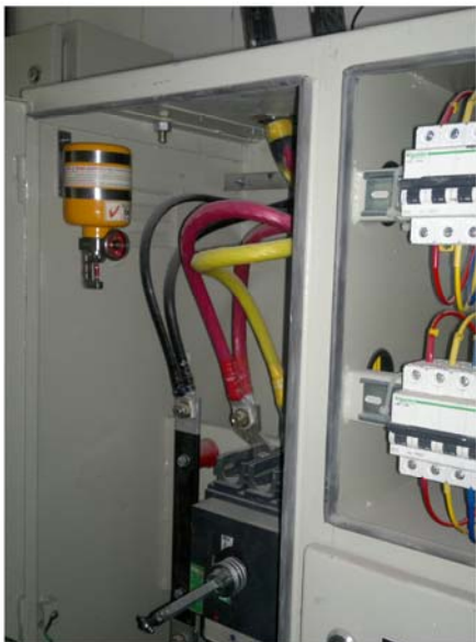
typical NASA 2T installation inside electrical panel
