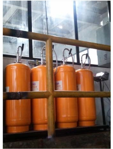
typical NASA fire suppression system for fire safety of a color coating unit
