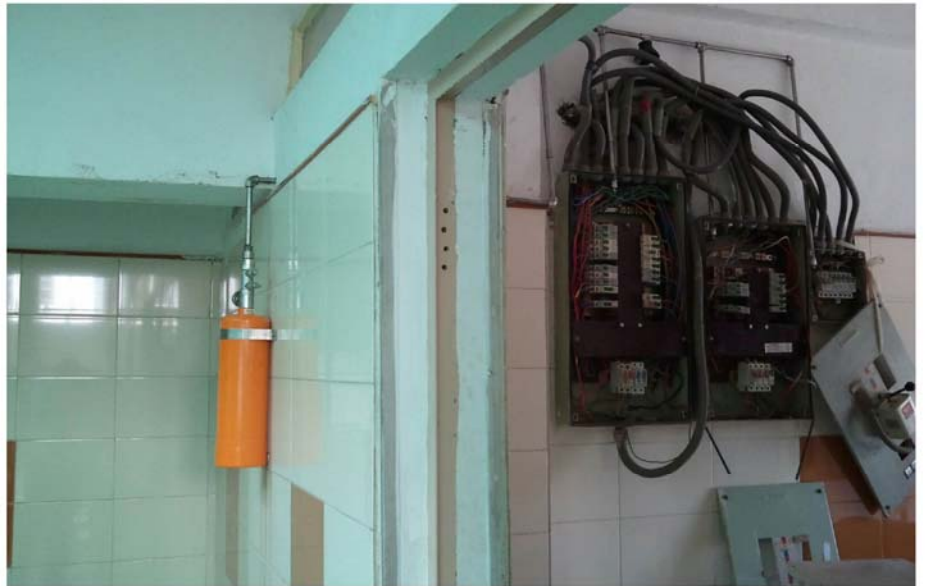
typical NASA fire suppression system for safety of electrical panels (in open condition)
