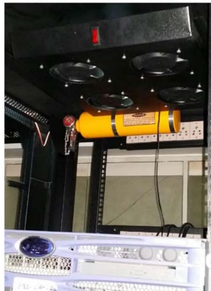
typical NASA 16T installation inside server rack
