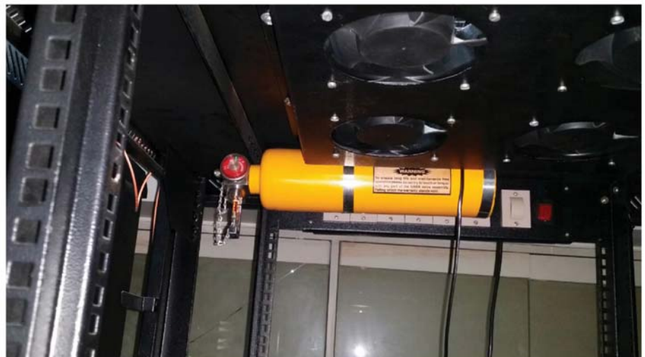
typical horizontal model installation inside server rack
