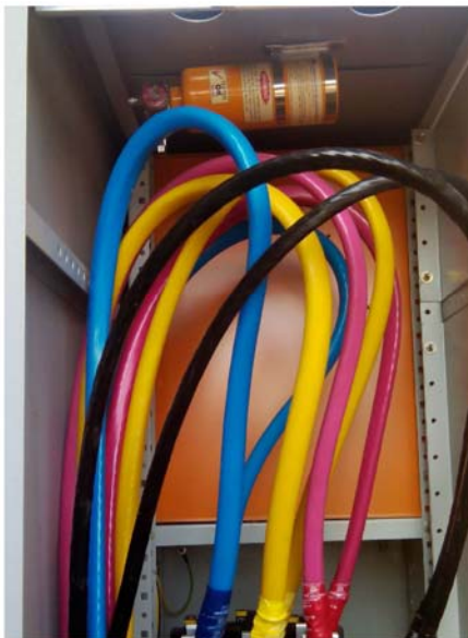
typical NASA 8T installation inside electrical panel
